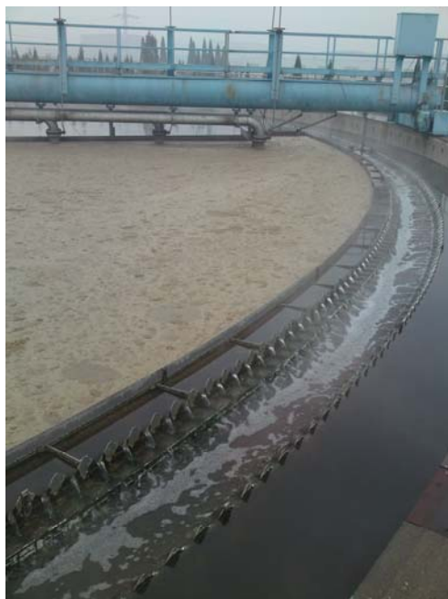
China Everbright International's sewage clarification basin in Jinan
